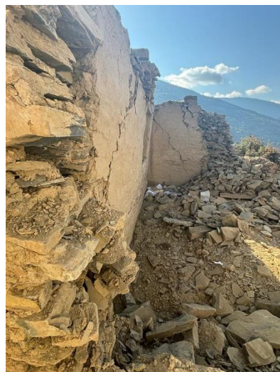
Figure 8. Destroyed Building of Shree Sita Mavi Barakot School, Jajarkot.
