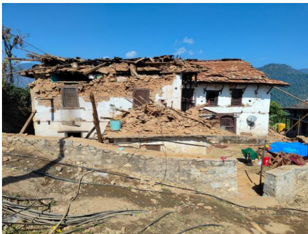
Figure 11. Bheri municipality community building after the earthquake.
