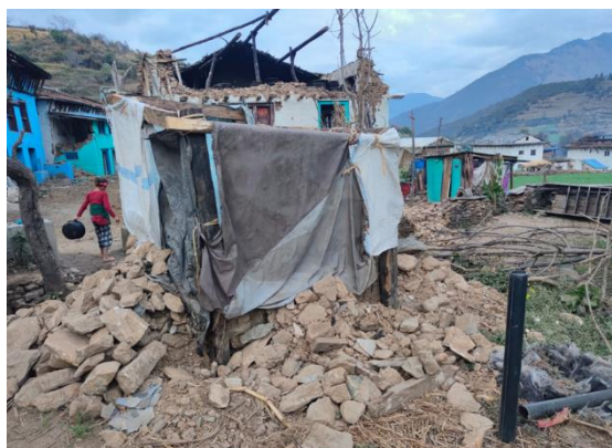
Figure 12. A toilet after the earthquake at Barekot Rural Municipality Ward No. 1, Shilpachaur.
