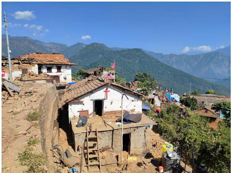
Figure 1. The damage caused by the earthquake to the religious places in Bheri Municipality, Ward No.3.
