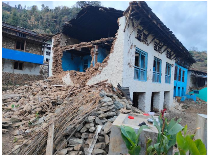
Figure 2 Destroyed Shilpachaur community building of Berekot rural municipality Ward No.1.
