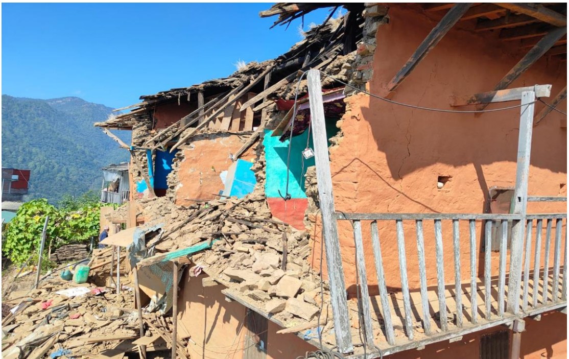
Figure 4. The damaged house by earthquake of Mr. Shambhu Chand of Bheri Municipality Ward No.3
